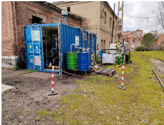
Figure 18. Decontamination module. Valladolid.
