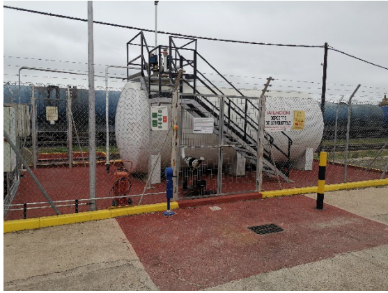
Figure 38. Zafra fuel supply facility
