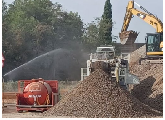
Figure 12. Ballast screening. A sprinkler irrigation system has been installed to minimise dust emission
