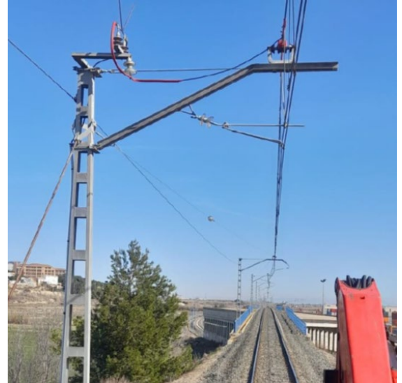
Figure 28. Anti-electrocution devices installed after an incident on the Madrid-Zaragoza-Portbou line
