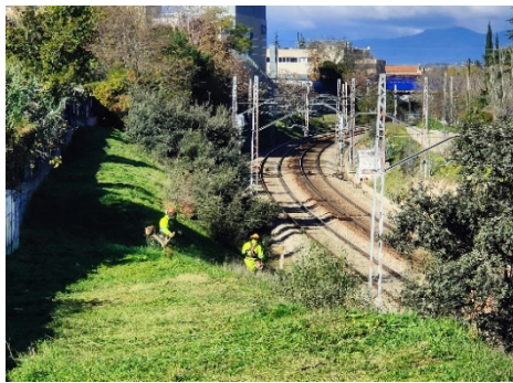
Figure 25. Fire protection measures on trackside
